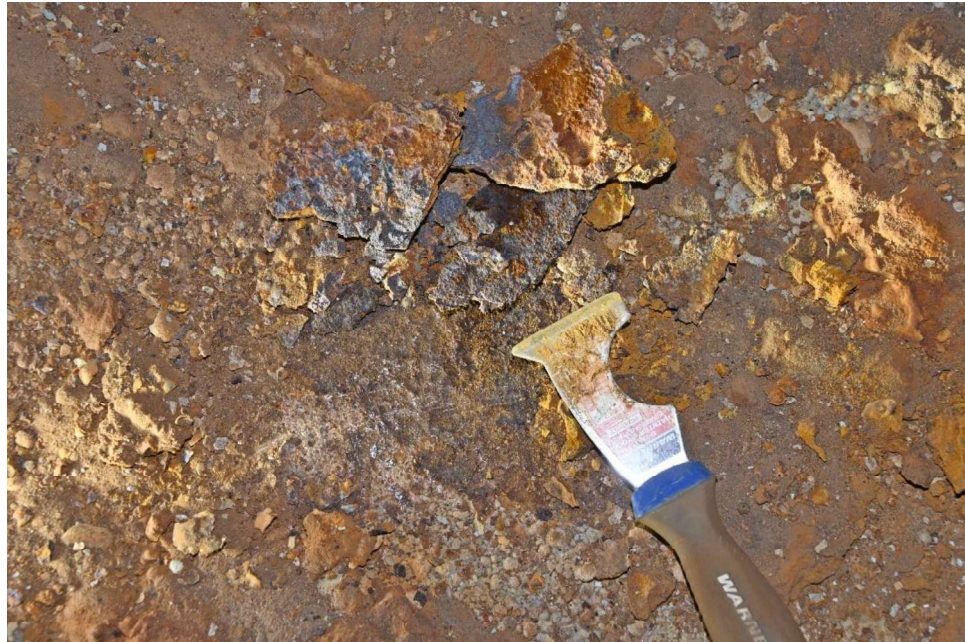
I-30 Close-up view of the bottom, illustrating rust scale that has been removed to examine the substrate. Note moderate to severe pitting is present in this area.
