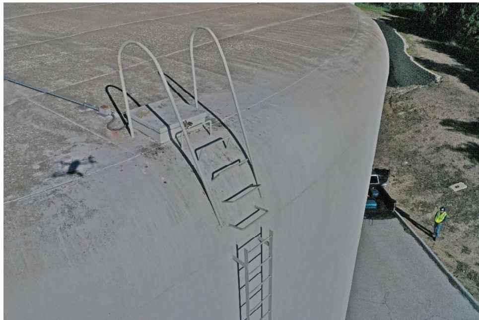
E-14 View of the top of the ladder, illustrating severe oxidation and fading and otherwise generally good condition of the paint system.
