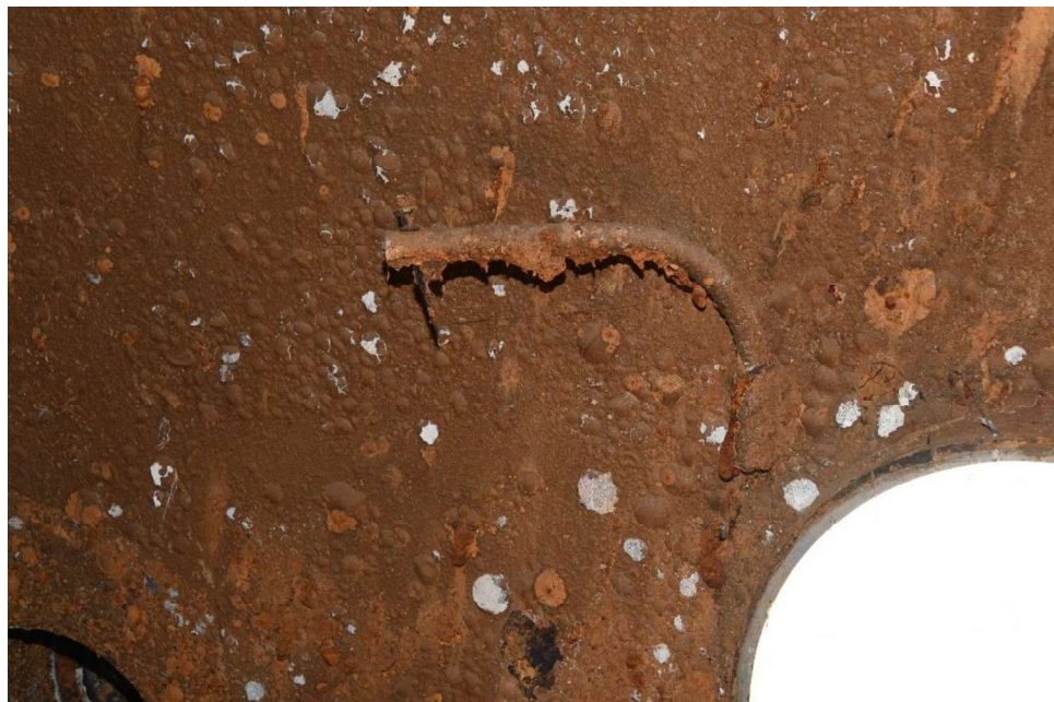
I-19 View of the manhole davit arm, illustrating a severely corroded davit arm and blistering and corrosion on the adjacent shell.
