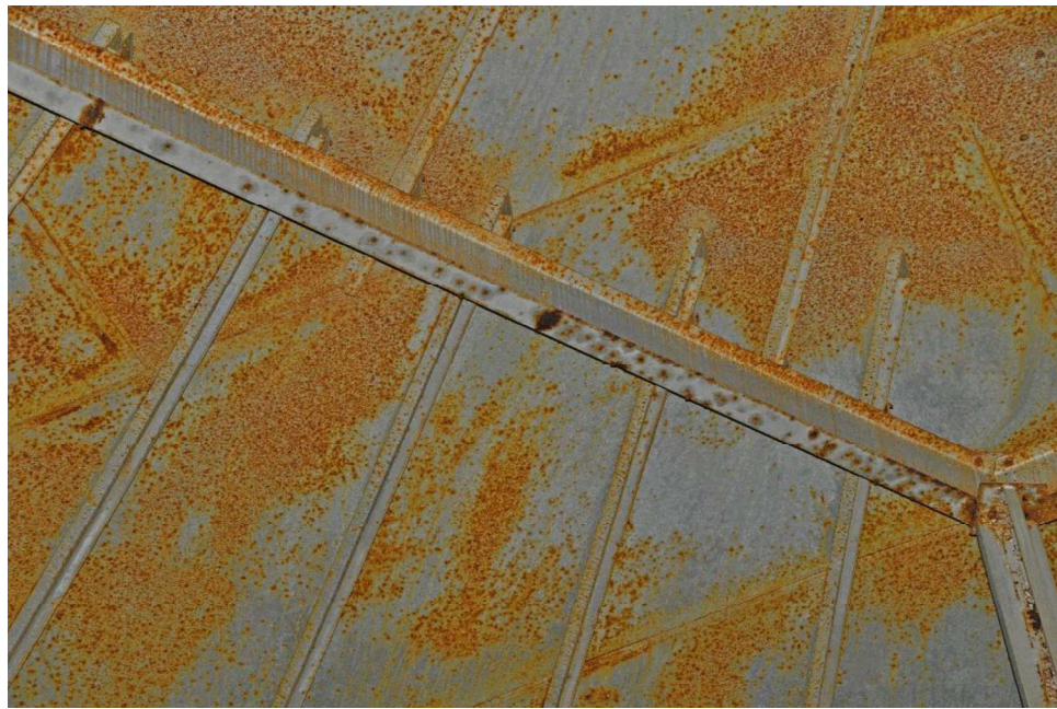
I-8 View of a girder, illustrating minor to moderate corrosion on the girder web and flanges.
