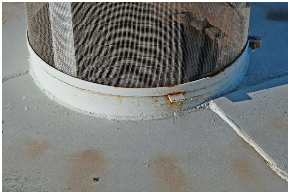
E-4 Same as Photo E-3, except a closer view of the vent neck.
