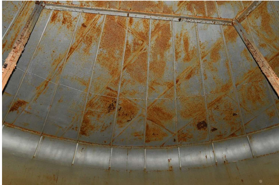
I-6 View of a portion of the outer bay, illustrating moderate to severe general corrosion on the roof and minor corrosion on the rafters.
