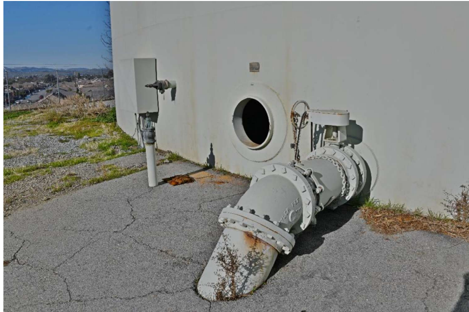
E-24 View of the inlet/outlet, illustrating random minor corrosion on the pipe, flanges, and valve actuator.
