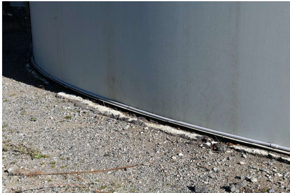
E-27 Same as Photo E-26, except in a different location. Note large gap under the tank in this location.
