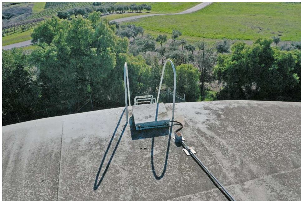
E-12 View of the roof hatch, illustrating severe oxidation and fading of the visible portion of the paint system.
