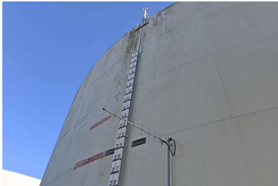
E-20 View of the LLI gauge board, illustrating minor fading of the numbering on the gauge board. Note top portion of the gauge board is missing.
