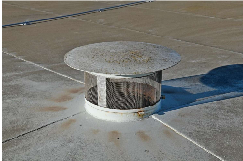
E-3 View of the center vent, illustrating minor corrosion on the vent cover and brackets.
