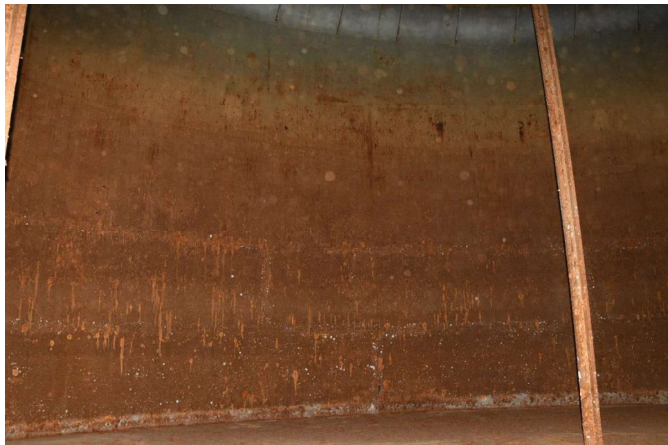
I-16 View of a portion of the shell, illustrating a layer of corrosion on all surfaces with random large rust tubercles present.
