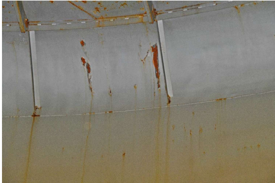
I-12 View of knuckle plates, illustrating delaminating topcoats with exposed prime coat present.
