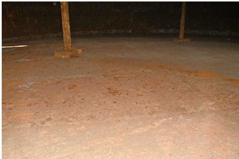
I-28 View of the bottom, illustrating moderate to severe corrosion on all surfaces.
