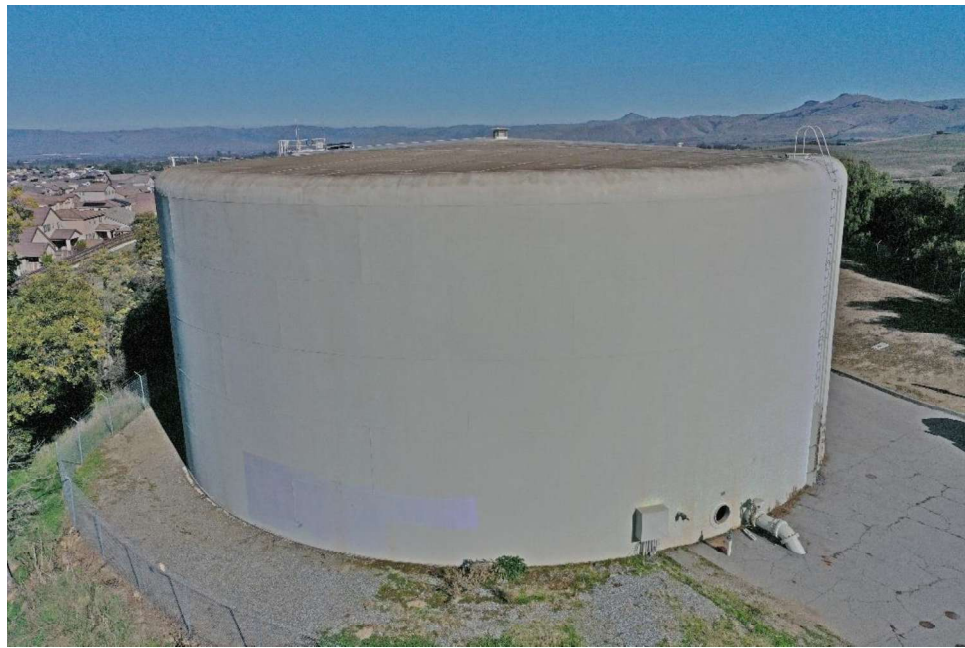
E-17 Same as Photo E-16, except in a different location. Note paint patchwork on the lower shell.
