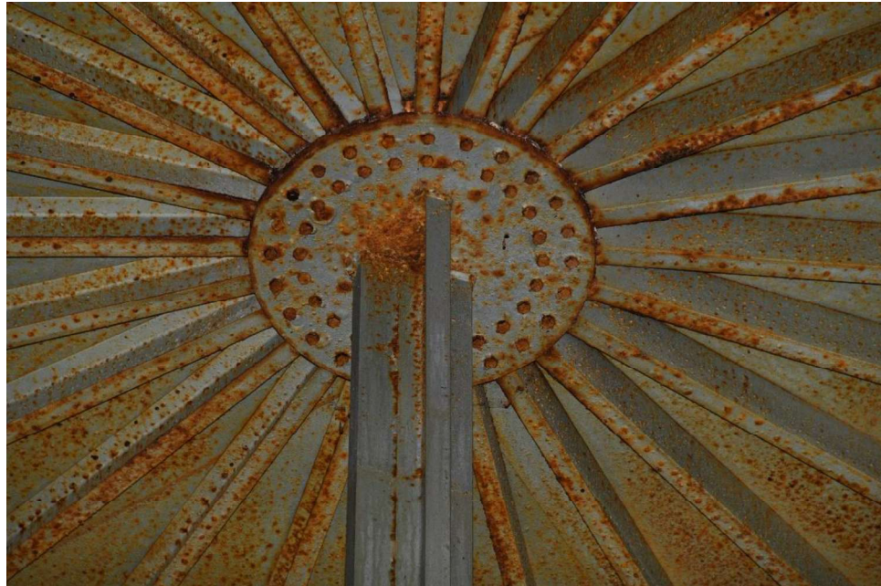
I-3 View of the center support plate, illustrating blistering of the silver coating system with minor to moderate corrosion on all surfaces.
