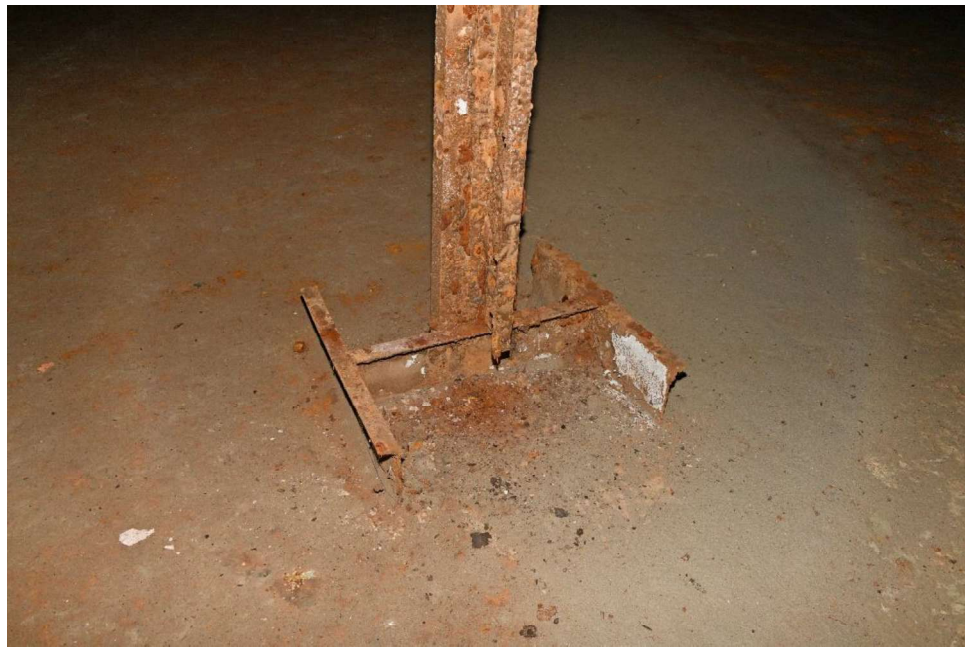
I-26 View of a column base, illustrating blistering, delaminating coating, and corrosion on the column and channel base.
