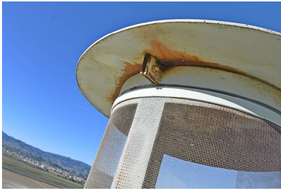
E-5 View of the underside of the center vent cover, illustrating moderate corrosion on the vent cover and brackets.
