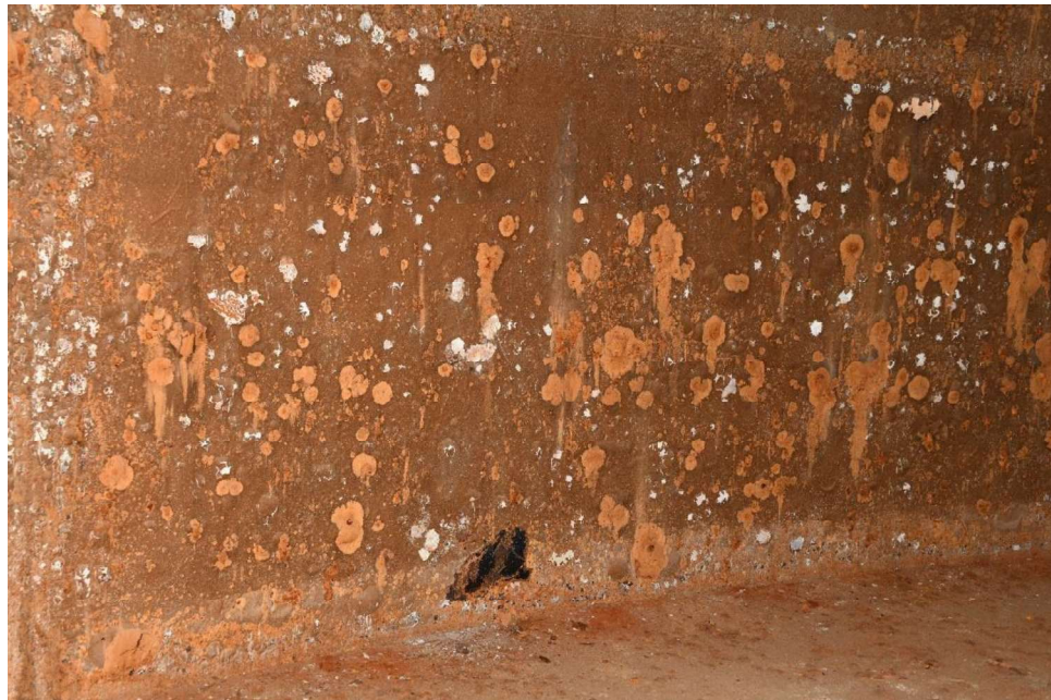
I-22 View of the shell to bottom transition, illustrating blistering, corrosion, and large rust tubercles on all surfaces.
