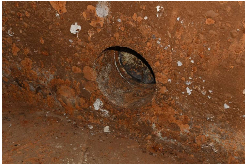
I-20 View of the inlet/outlet, illustrating blistering and corrosion on all surfaces.
