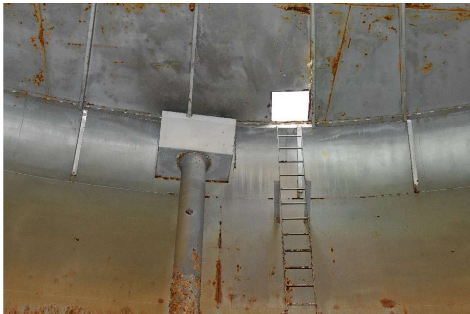
I-13 View of the roof hatch and overflow, illustrating moderate to severe corrosion along the edges of the roof hatch curb, overflow weir box and pipe, and ladder.
