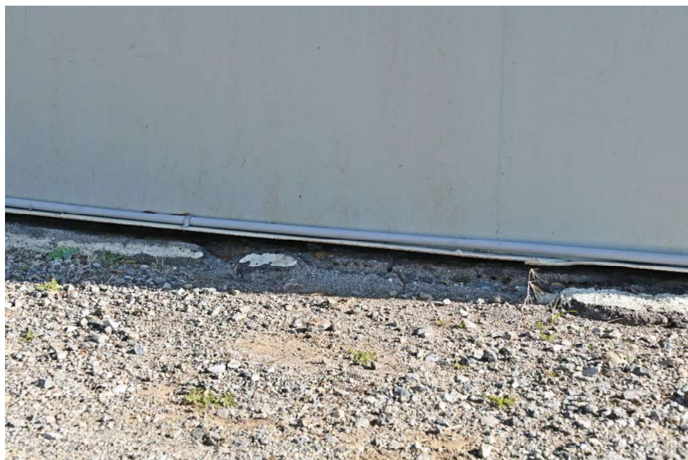
E-28 Same as Photo E-27, except a closer view of the gap under the tank.
