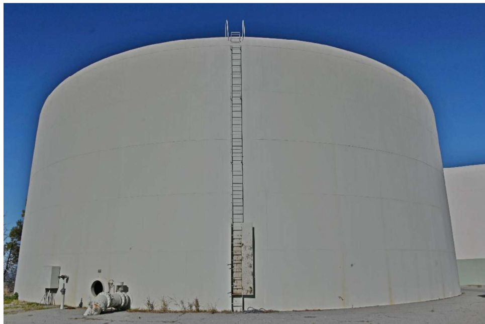
E-16 View of a portion of the shell, illustrating moderate to severe oxidation and fading and otherwise generally good condition of the paint system.
