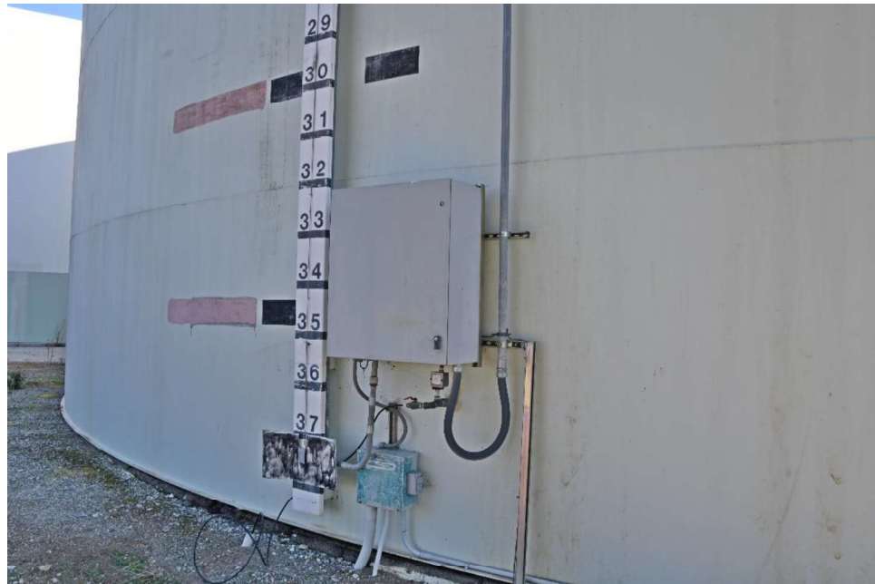
E-21 Same as Photo E-20, except at the bottom of the LLI gauge board. Note fair to good condition of the adjacent equipment boxes and conduit.
