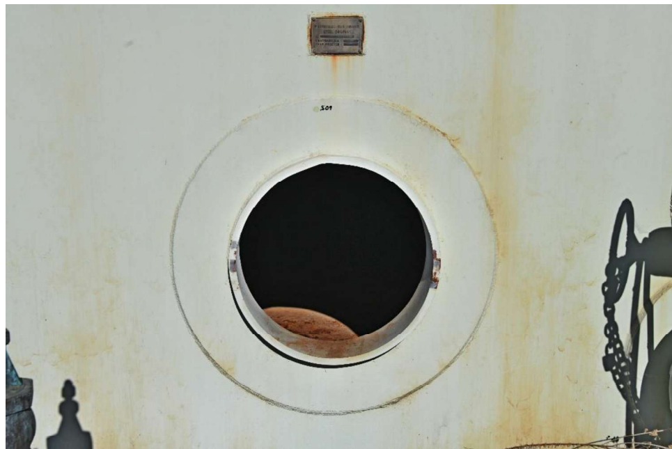
E-22 View of the manhole, illustrating mechanical damage with minor corrosion on the stiffener ring and staining on the adjacent shell.
