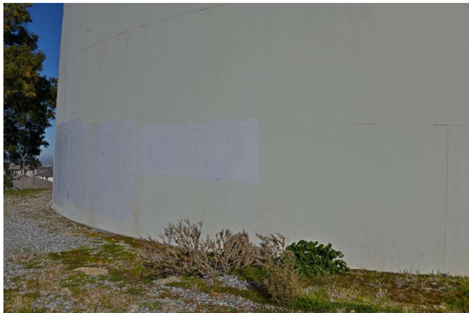
E-19 View of the lower shell, illustrating an area of paint patchwork. Note generally good condition of the adjacent paint system.
